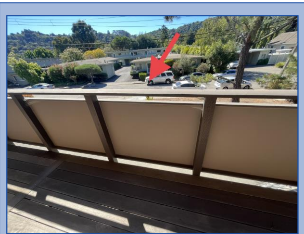
Railing is loose; repairs are recommended
