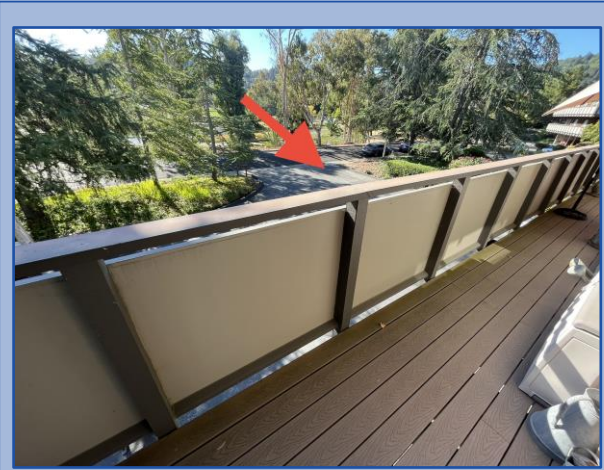
Railing is loose; repairs are recommended
