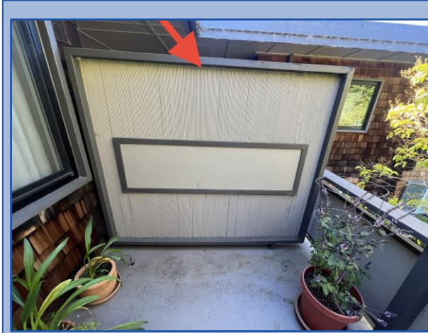
Separation wall is loose; repairs are recommended
