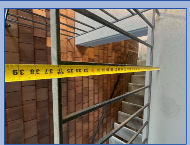
Railing height and baluster spacing do not meet current building code requirements
