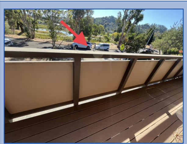
Railing is loose; repairs are recommended
