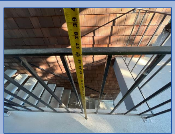
Railing height and baluster spacing do not meet current building code requirements
