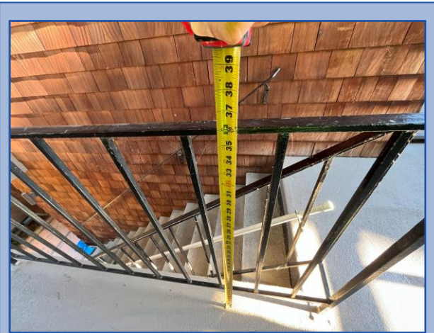
Railing height and baluster spacing do not meet current building code requirements
