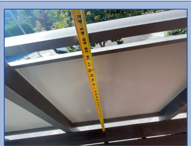
Railing height does not meet current building code requirements
