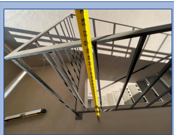
Railing height and baluster spacing do not meet current building code requirements
