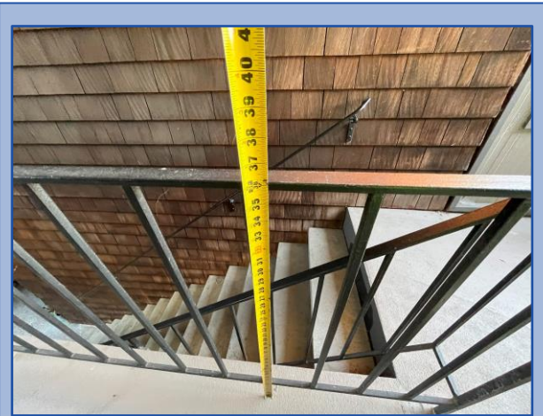
Railing height and baluster spacing do not meet current building code requirements
