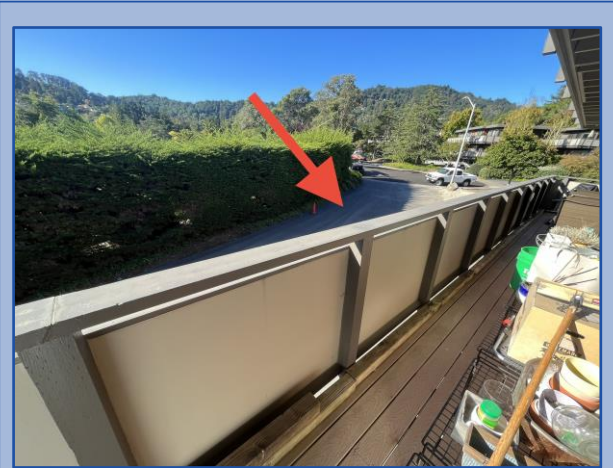
Railing is loose; repairs are recommended
