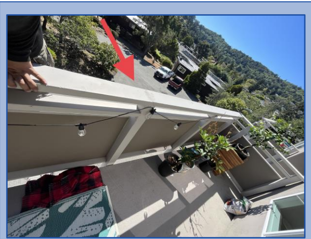
Railing is loose; repairs are recommended
