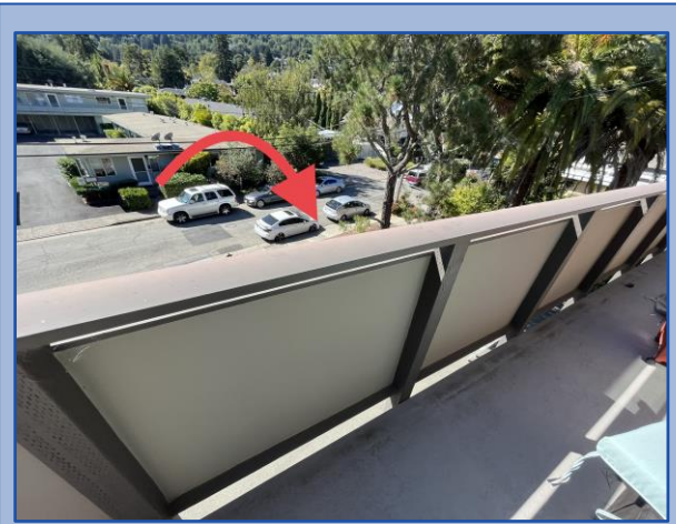
Railing is loose; repairs are recommended
