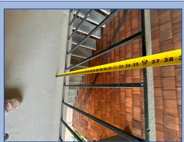
Railing height and baluster spacing do not meet current building code requirements
