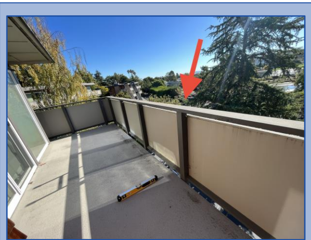
Railing is loose; repairs are recommended
