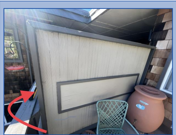
Loose and decayed separation wall; repairs are recommended
