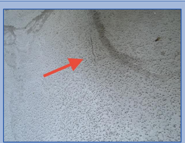
Balcony surface contains small crack; repairs are recommended
