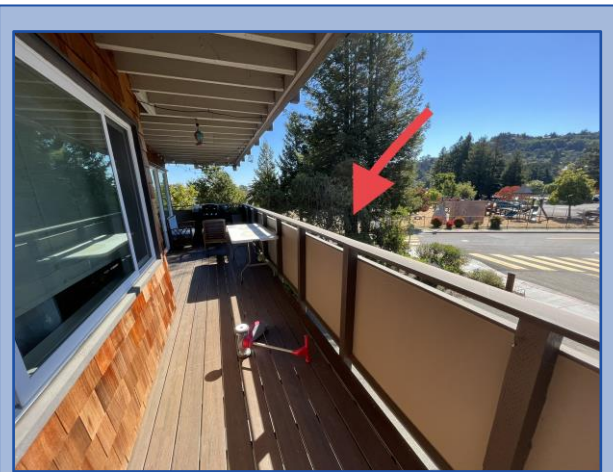
Railing is loose; repairs are recommended
