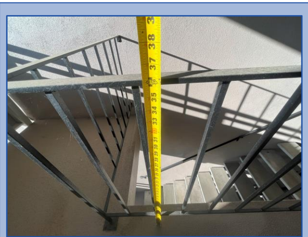
Railing height and baluster spacing do not meet current building code requirements
