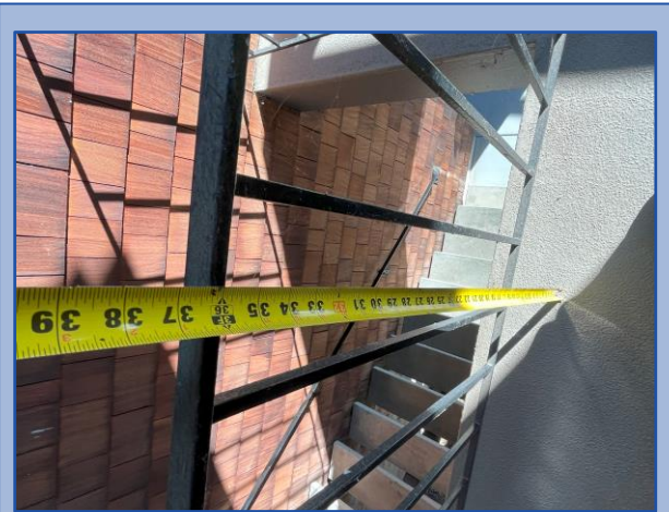
Railing height and baluster spacing do not meet current building code requirements
