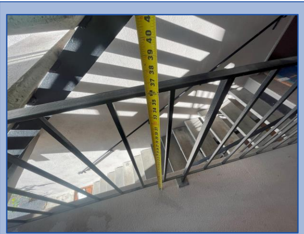
Railing height and baluster spacing do not meet current building code requirements
