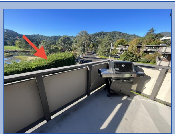
Railing is loose; repairs are recommended
