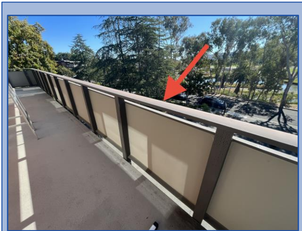
Railing is loose; repairs are recommended
