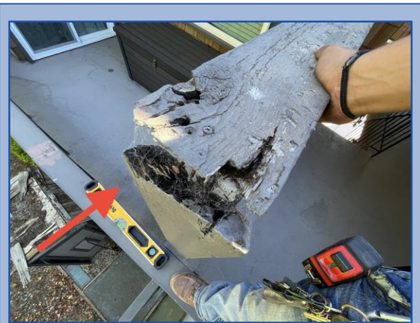
Rotted and loose separation wall; repairs are recommended
